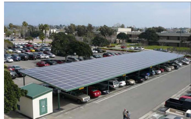
Naval Base San Diego Solar carport (57 KW)
